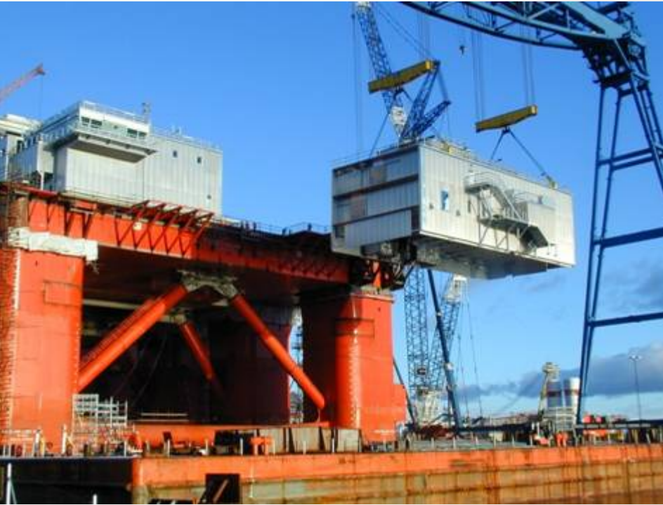
H6e LQ Spitsbergen Installation
